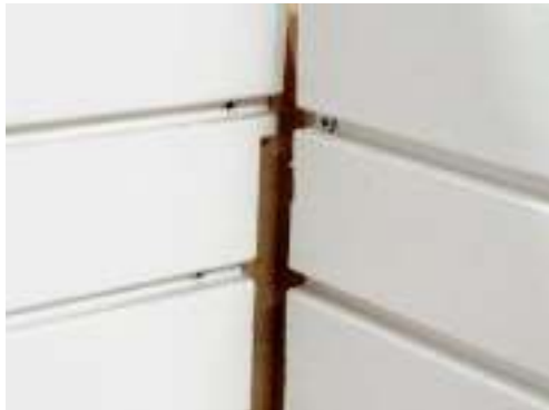
PANEL ENDS CAN BE UNEVEN
